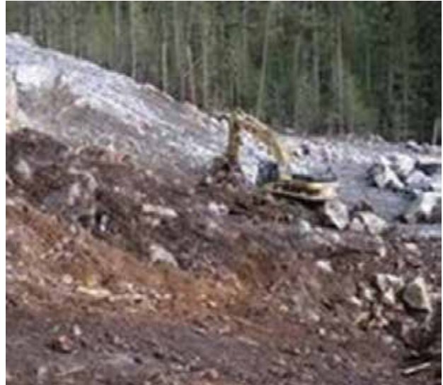
Before Sam Fitzpatrick was killed by a boulder, concerns had been expressed to Kiewit management about excavator work being performed above workers.
